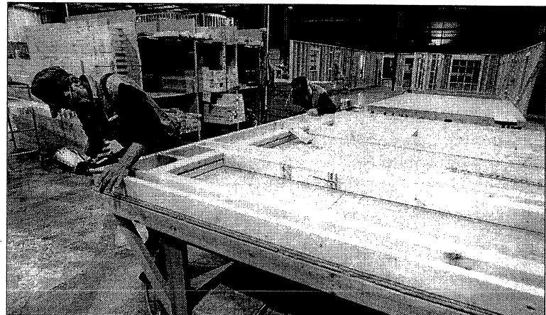
Carpenters Bob Moore, left, and Glenn Kaufman are building a wall at the New Hope Construction warehouse in Hendersonville. The wall is for a house that will be shipped to Bedford County, Va., for a low-income family. The nonprofit organization also is building housing for hurricane victims in Hancock County, Miss.
